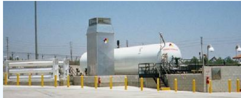
Tank, pumps, vaporizer, containment, buffer
