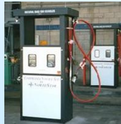
Fueling island dispensers
